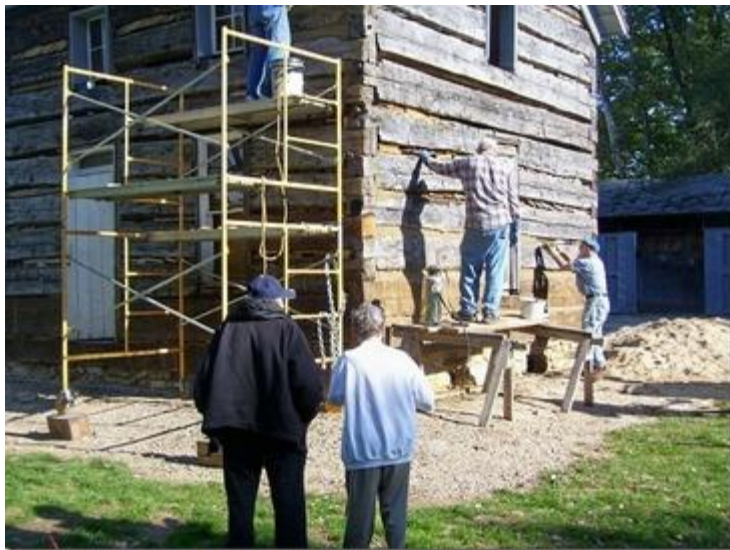
Long-time volunteers, Bill and Pat Draper, watch as the MWF crew works on filling the space between the logs.
