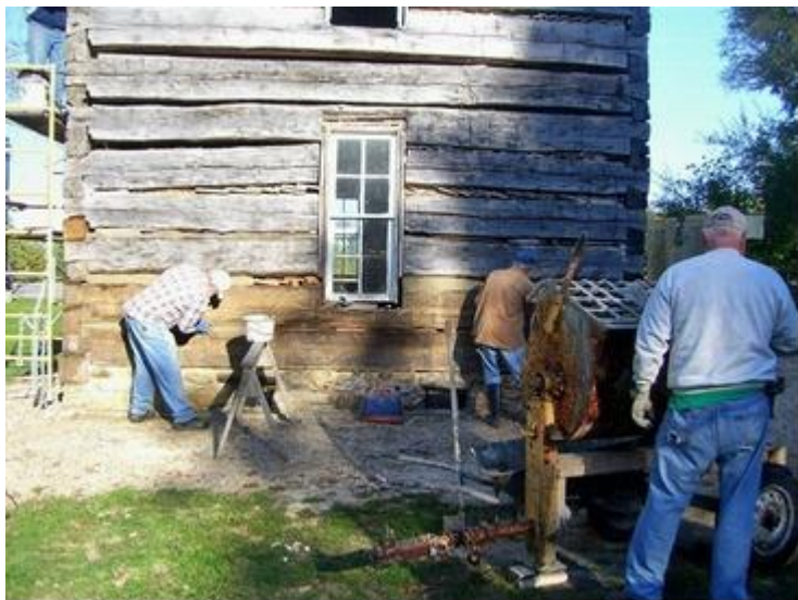
Vern Cripe mixes mortar as the MWF crew tackles the process of "chinking" to fill the spaces between logs.
