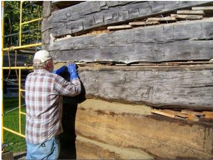
Al Auffart chinks between logs on the Fouts Home. Notice the blocks of wood that are wedged into the space between logs, then covered with the "mud."
